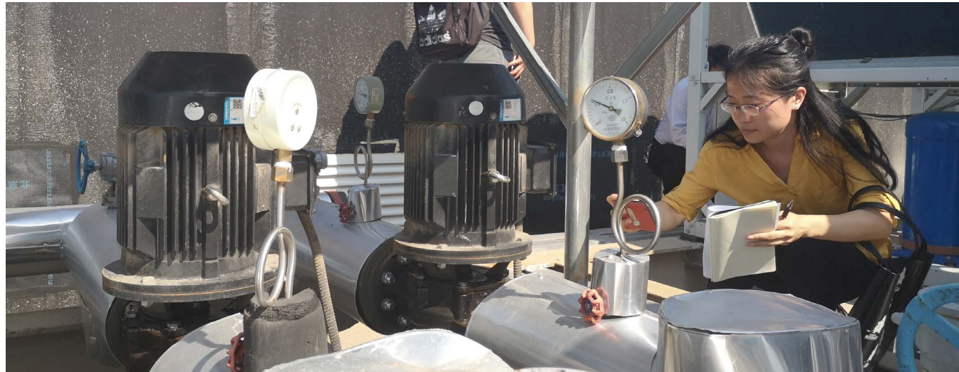
Photo: Energy audit at Beijing Ditan Hospital, China
