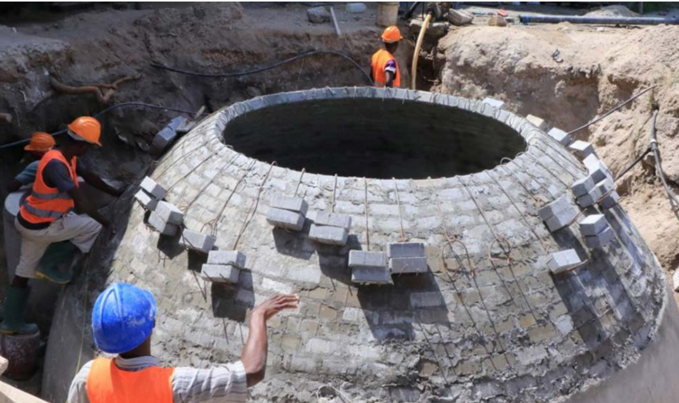
Photo: Construction of biodigestion facility for health care waste, Dar es Salaam, Tanzania
