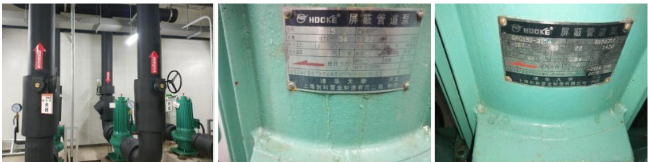
Photographs and nameplates of circulating water pumps
