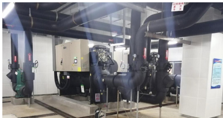
External view of ground-source heat pump system
