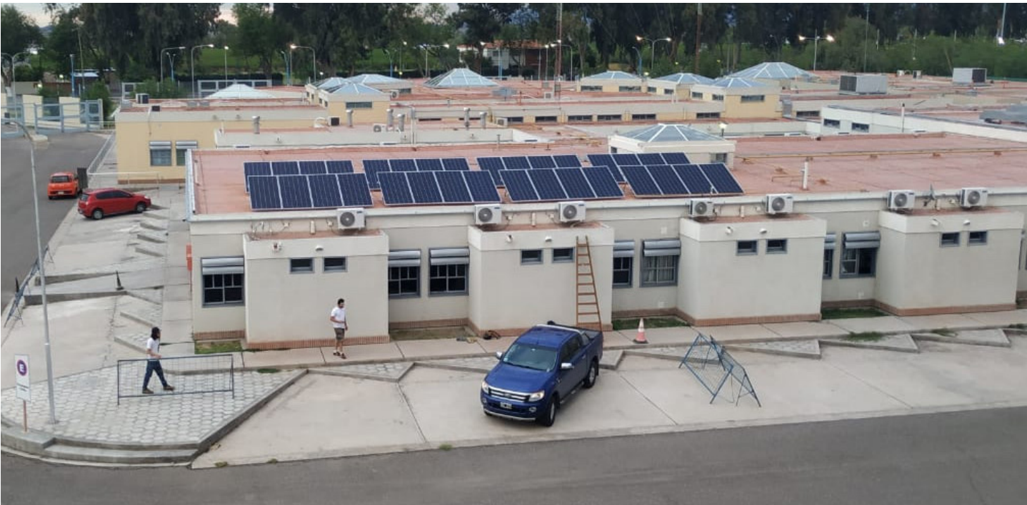
Photovoltaic panels (solar energy) installation in Dr. J. Giordano Hospital. San Juan, Argentina
