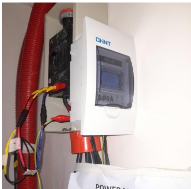
Ongoing power consumption monitoring
