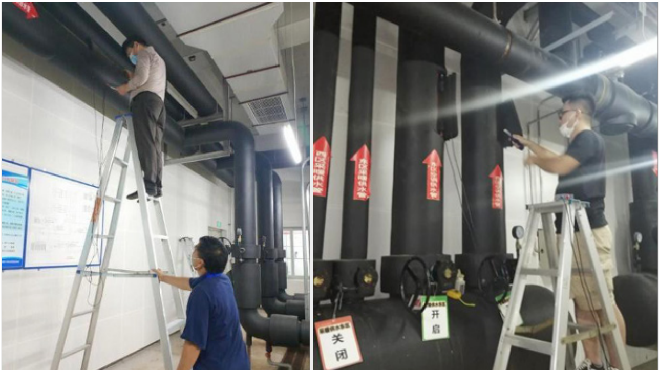
Field collection of air conditioning and ground source side supply and return water flowrate
