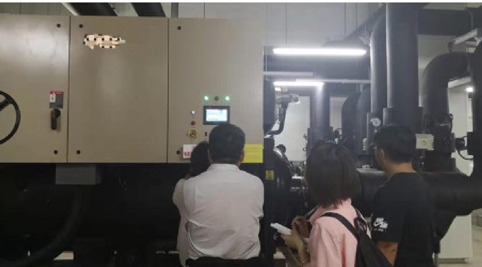
Observing mechanical equipment during the cooling audit at Beijing Huilongguan Hospital
