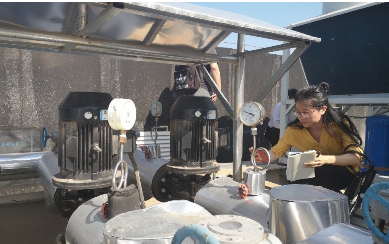
Evaluating roof-top equipment during the cooling energy audit at Beijing Ditan Hospital.
