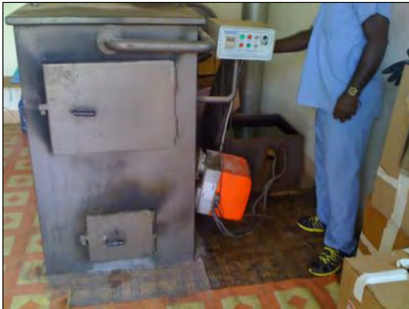
Chinese incinerator that does not meet international standards (used for sharps)
