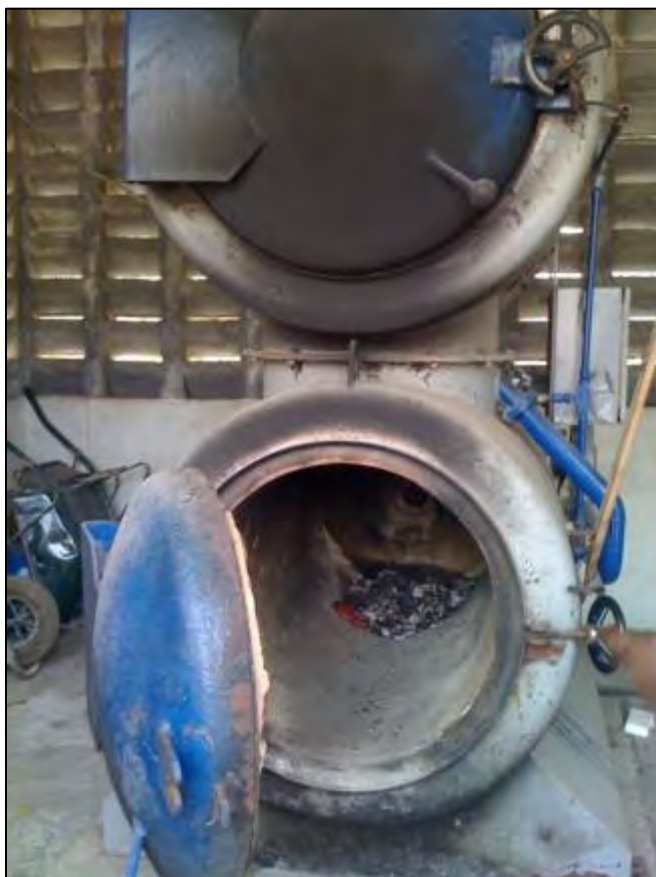
Broken incinerator that does not meet international standards
