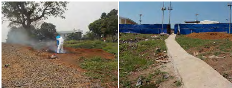
Figure 9. Left - worker manually dumping Ebola-contaminated waste into the burn/burial pit in the green zone of the hospital (note residences and residents in the background and the potential for wind to blow away some of the waste); Right - photo showing the distance between the red zone in the background and the location of the burn/burial pit from where the photo was taken at an ETU
