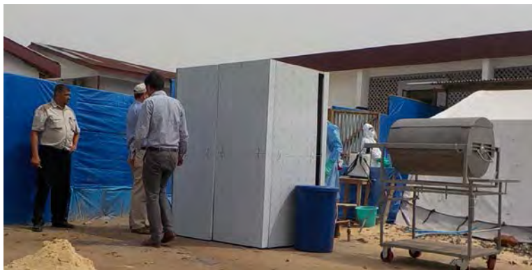
Figure 22. First autoclave unit during installation at No. 34 Hospital, Freetown, Sierra Leone
