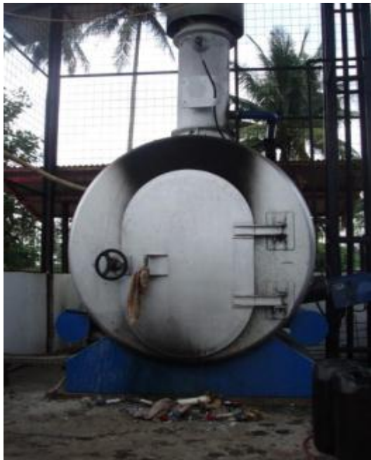
A typical medical waste incinerator, showing stains where black smoke leaks from the primary combustion chamber, and unburned waste scattered on the floor. Most medical incinerators are operated below 600o C and feed by diesel fuel lead to high cost medical wastes operations. (@Balifokus)
